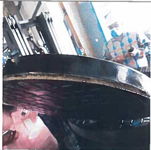
FOUND CRACK ON COVER PLATE (DN-1000 mm)
