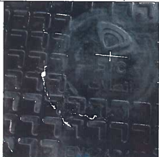
FOUND CRACK ON COVER PLATE (DN-1000 mm)
