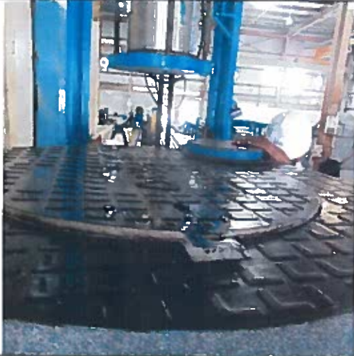
FOUND CRACK ON COVER PLATE (DN-1000 mm)
